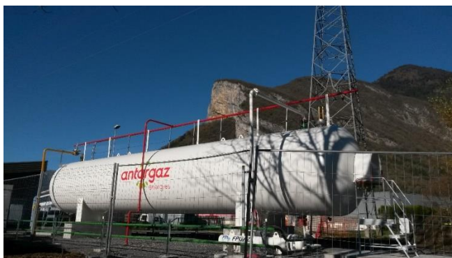
Cuve propane 70 m3 _ 31 Tonnes
